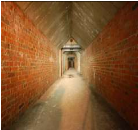
One of the corridors in the Deep Shelter. The ceiling, walls and floor appear to be in excellent condition, given that the Shelter was closed and sealed in 1944.
